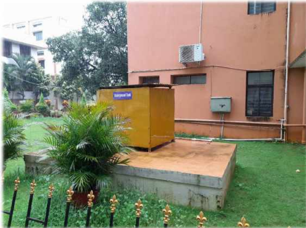
Underground water tank
