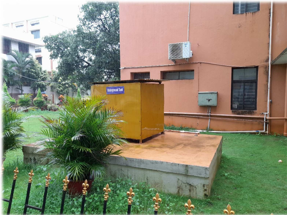
Underground water tank
