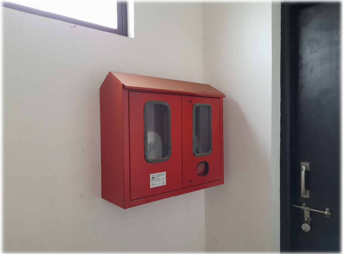
Firefighting hose pipe
