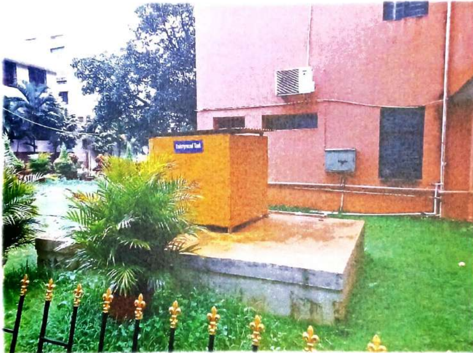
Underground water tank
